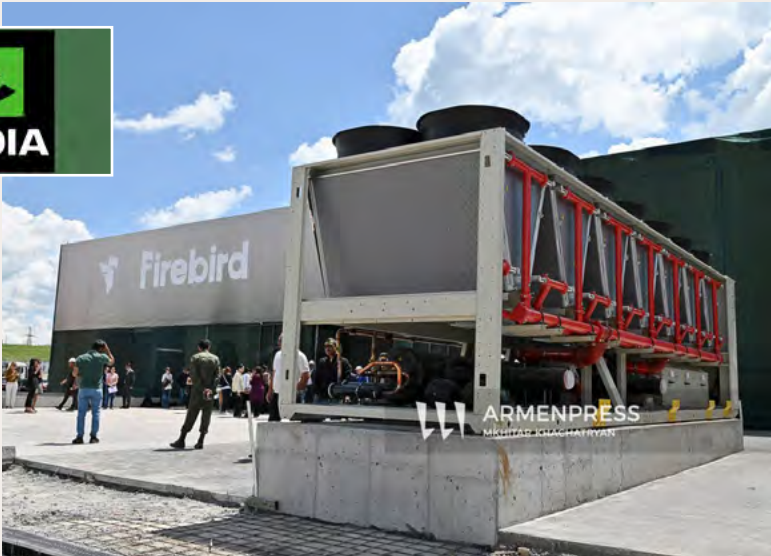
Firebird data center in Armenia
