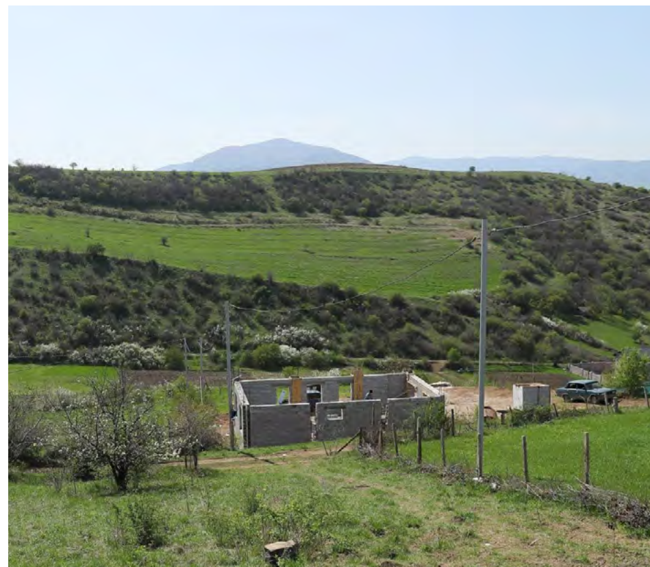
A new house is built in Berkaber, a border village in Tavush province, April 17, 2024.
