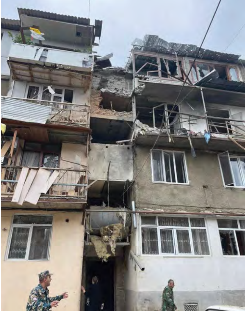
Destroyed apartment building in Stepanakert
