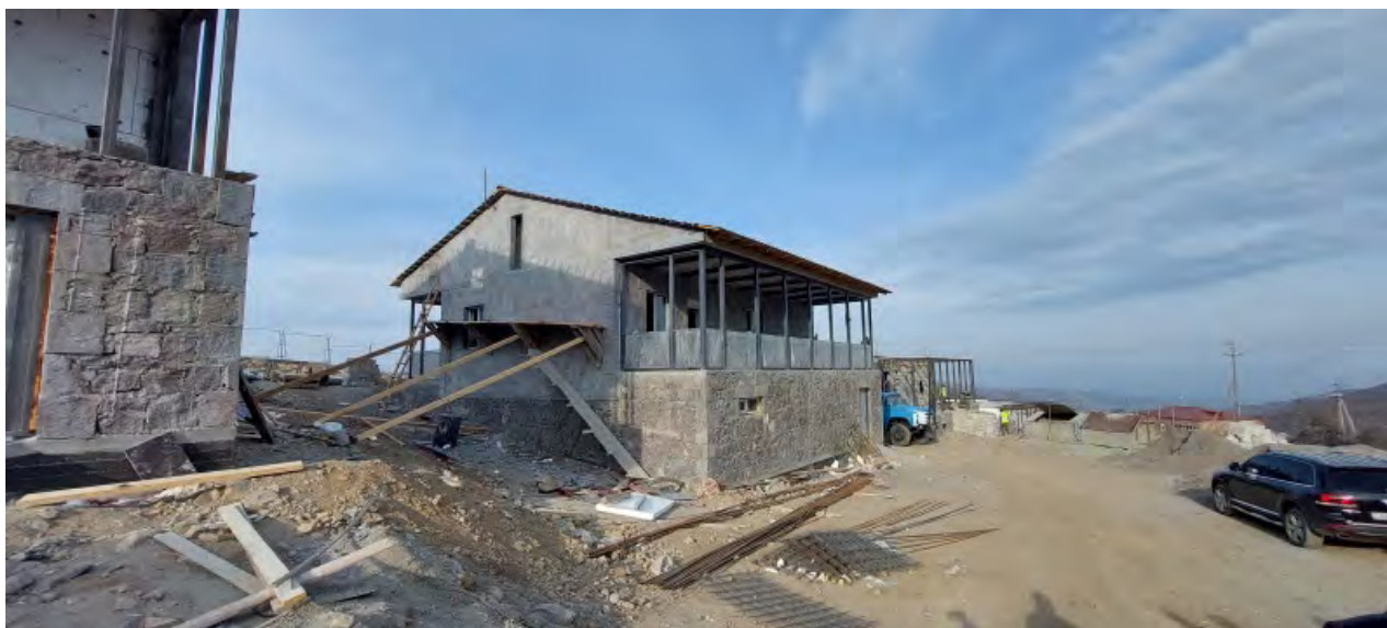
The construction of a new district in Shurnukh village, March 14, 2022. (Photo Armenian Urban Development Committee)
