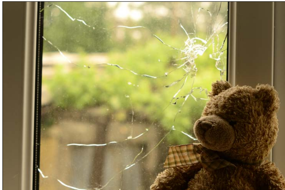
A window damaged in Tavush
