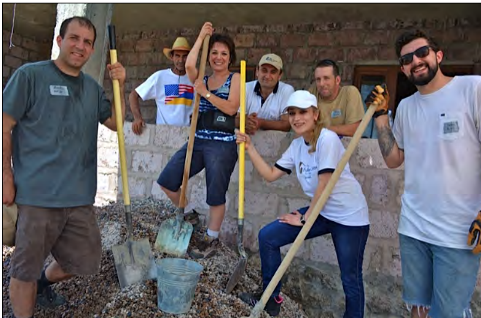
Team members, homeowner Archanik Simonyan (top left), and the Fuller Center staff get ready to prepare the concrete flooring.
